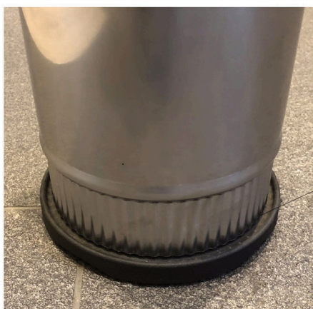
Flue seated correctly.
